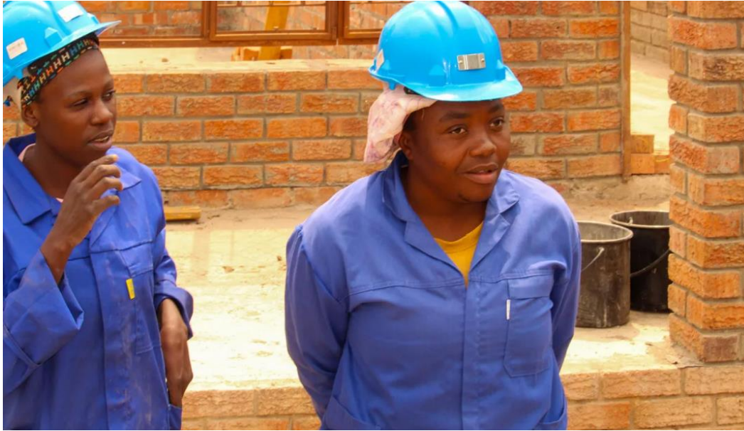
Nomathemba Sibanda displays her masonry skills at the public works site in Filabusi town, southern Zimbabwe. Photo: LWF/Monmo Dahiru Moodi https://lutheranworld.org/news/zimbabwe-new-hope-and-decent-work-home
